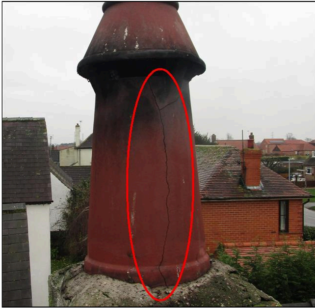
9.3 Item 3(Picture) Crack to the chimney pot
