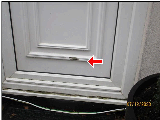
14.3 Item 5(Picture) Damage to the front door
