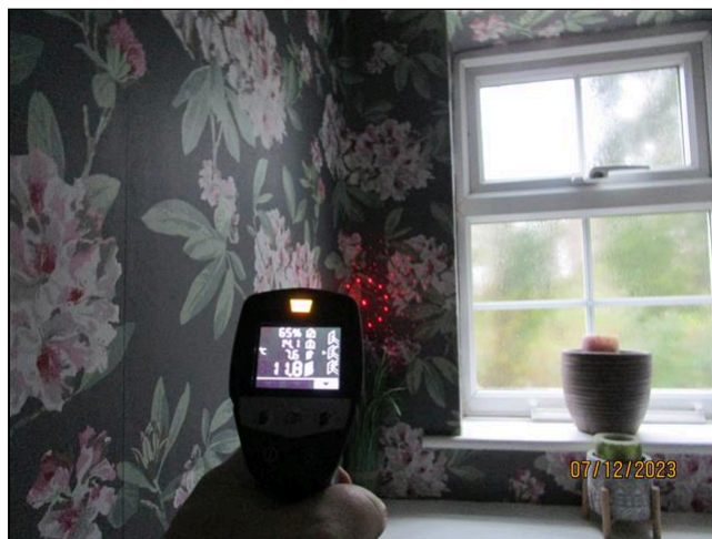
3.2 Item 4(Picture) Some elevated condensation readings
