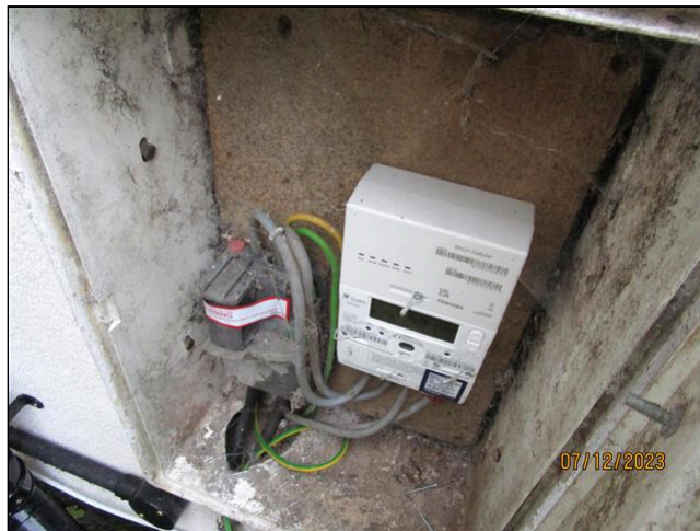
29.0 Item 2(Picture) Electric meter
