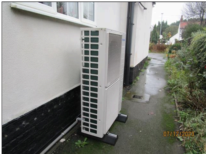
31.0 Item 2(Picture) Air source heat pump
