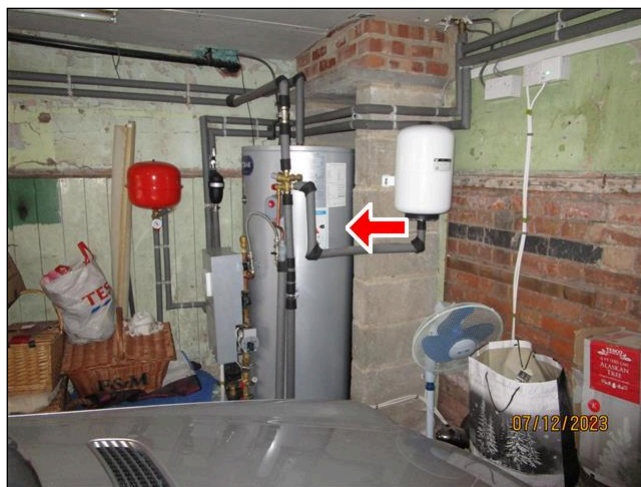
31.3 Item 2(Picture) New Hot Water Tank in the garage
