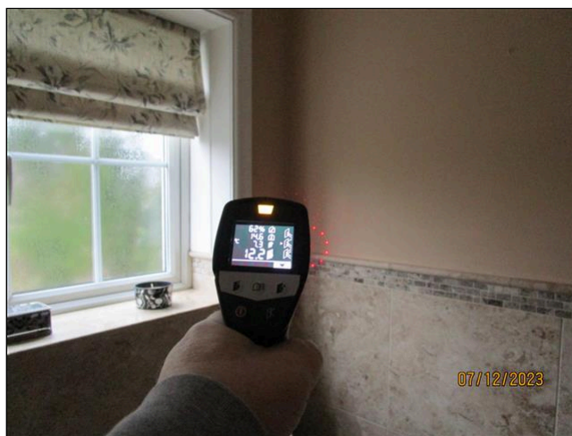
24.0 Item 2(Picture) Elevated condensation readings in Bathroom
