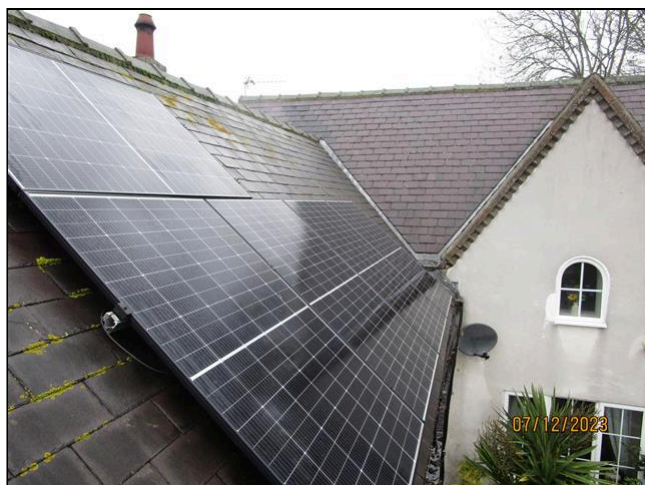
2.12 Item 1(Picture) PV Panels
