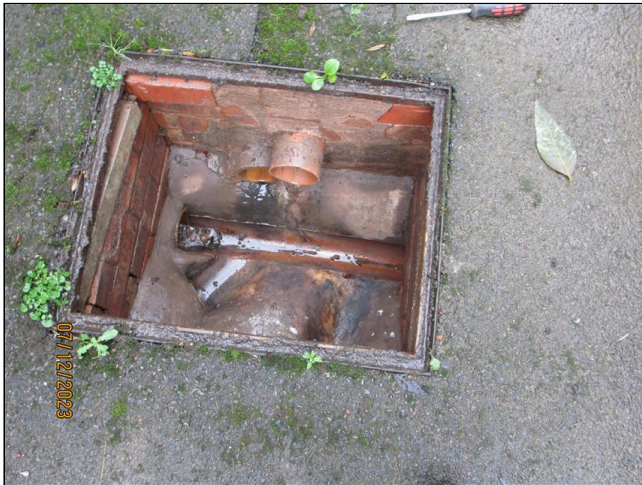
32.3 Item 1(Picture) Drain running clear
