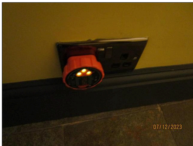
29.0 Item 3(Picture) Electric socket tests
