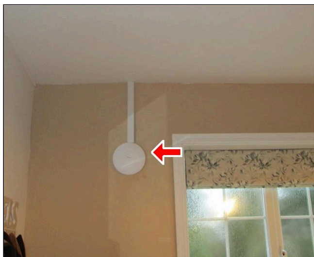
24.0 Item 1(Picture) Vent in the Bathroom was switched off
