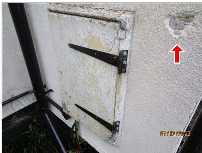
13.3 Item 3(Picture) Damage to wall render
