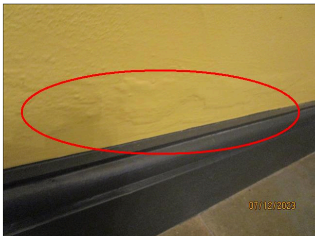
3.2 Item 3(Picture) Signs of damp at the base of the wall in Hall/Kitchen
