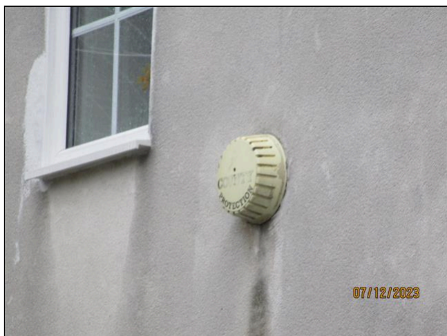
7.9 Item 1(Picture) Intruder alarm not tested
