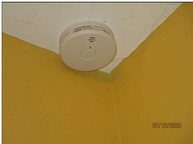
7.0 Item 1(Picture) Smoke alarm not tested
