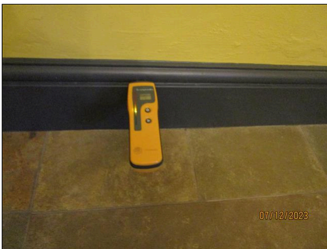
22.3 Item 3(Picture) Skirting checks
