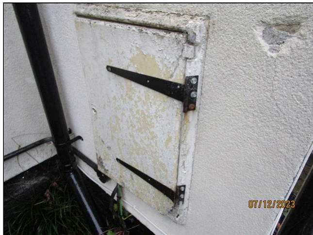
29.0 Item 1(Picture) Electric meter cabinet
