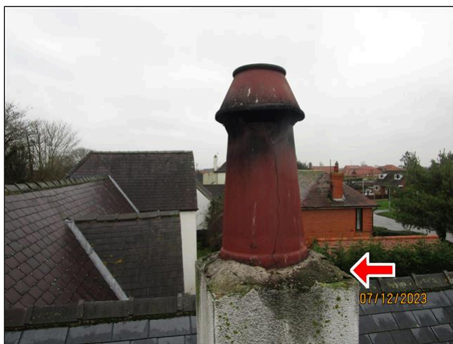
9.3 Item 1(Picture) Flaunching may have cracks
